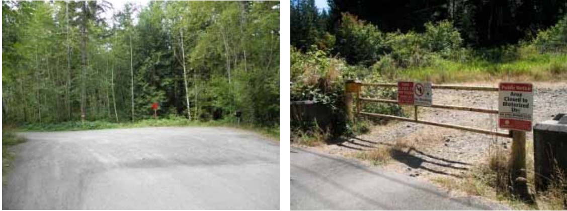
Figure 5-4: Dead end roads with insufficient turnaround space.
