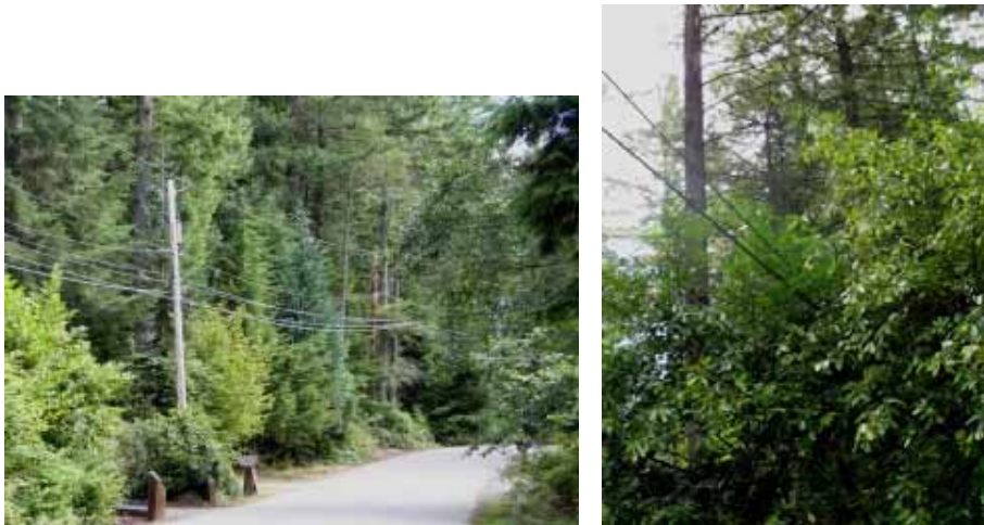
Figure 5-16: Above ground utilities are vulnerable to fire.
