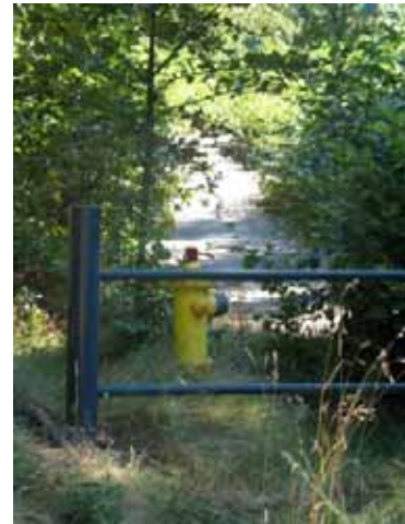
Figure 4-2: Fire hydrant at Sorenson Street (with vandal resistant lock).
