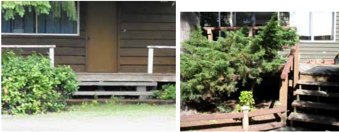
Figures 5-11: Lack of screening under porches and decks.
