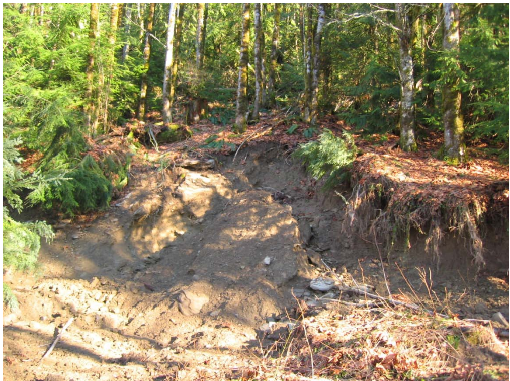
Figure 39 Cut slope slide. Photograph taken standing on CL-1000 Mainline Road. Photograph taken in January 2009. View looking east. (Photo by M. Penney)
