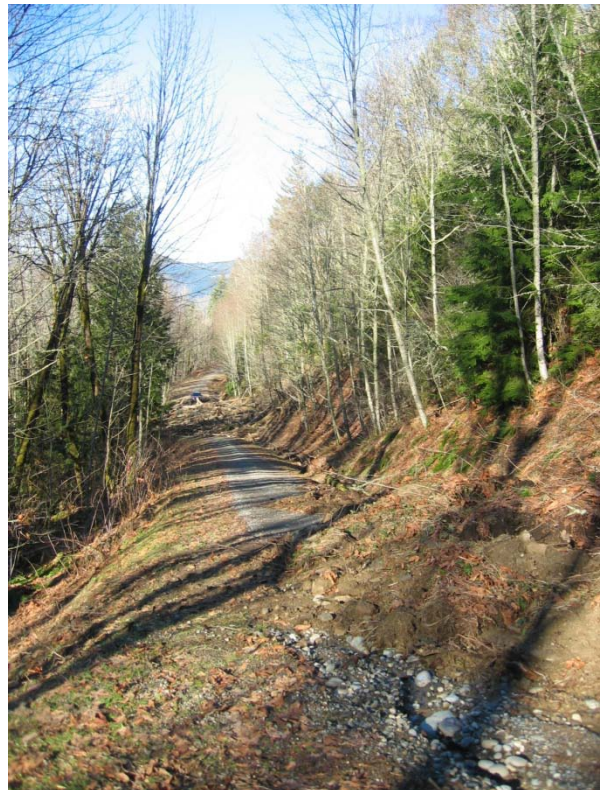
Figure 43 Channel eroded when water from inboard ditch was diverted by deposit from cut slope slide. Water was directed over outboard edge of road fill. Photograph taken in January 2009. View looking northwest. (Photo by M. Penney)
