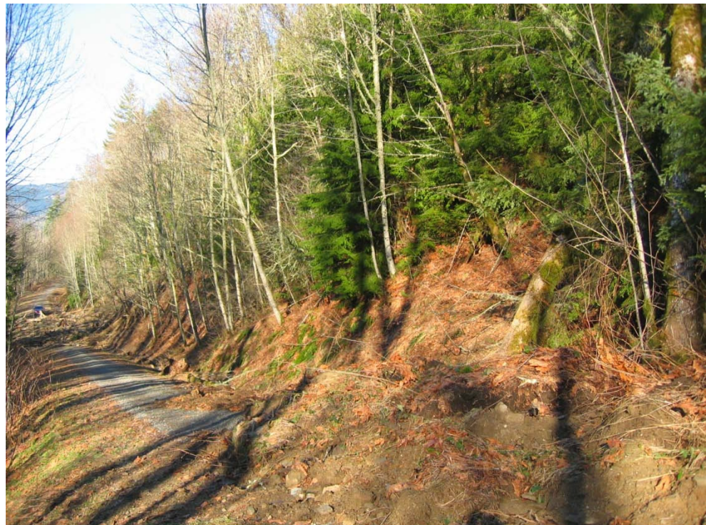
Figure 41 Slide debris from the cut slope slide deposited on the CL-1000 Mainline Road. Debris from Cliff Slide can be seen on road in background. Photograph taken January 2009. View looking north. (Photo by M. Penney)
