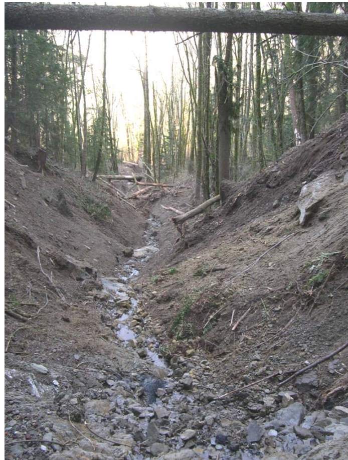
Figure 5 Scour of lower reaches of debris flow track at 3810 NR site. Photograph taken in Spring 2009. View looking northwest. (Photo by C. Hanell)
