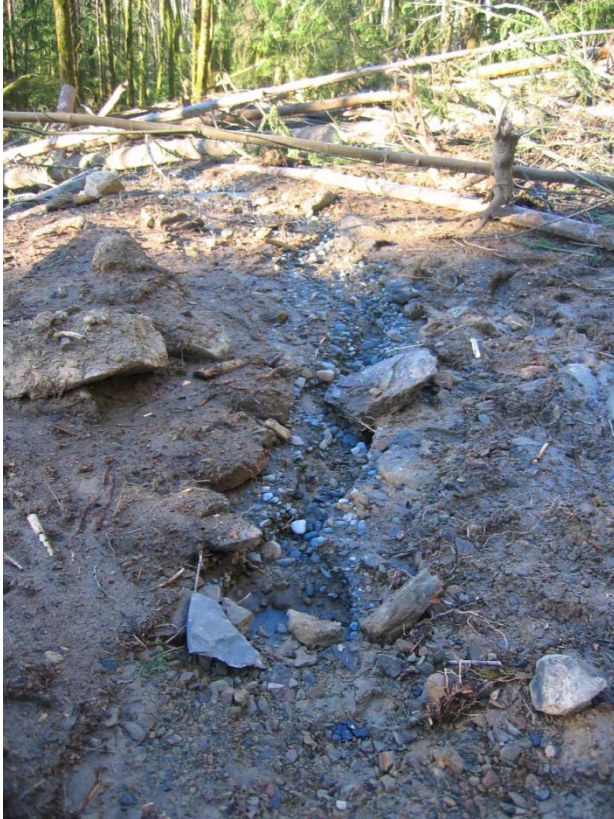
Figure 42 Diversion channel at Cliff Slide deposit. Water collected by slide debris diverted through the channel eroded along edge of slide debris and directed over outboard edge of road fill. Photograph taken in January 2009. View looking northwest. (Photo by M. Penney)
