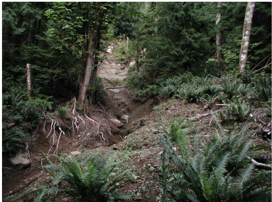
Figure 29 Scoured slopes and channel below Middle PI. Photograph taken Fall 2009. View looking easterly. (Photo by J. Coyle)
