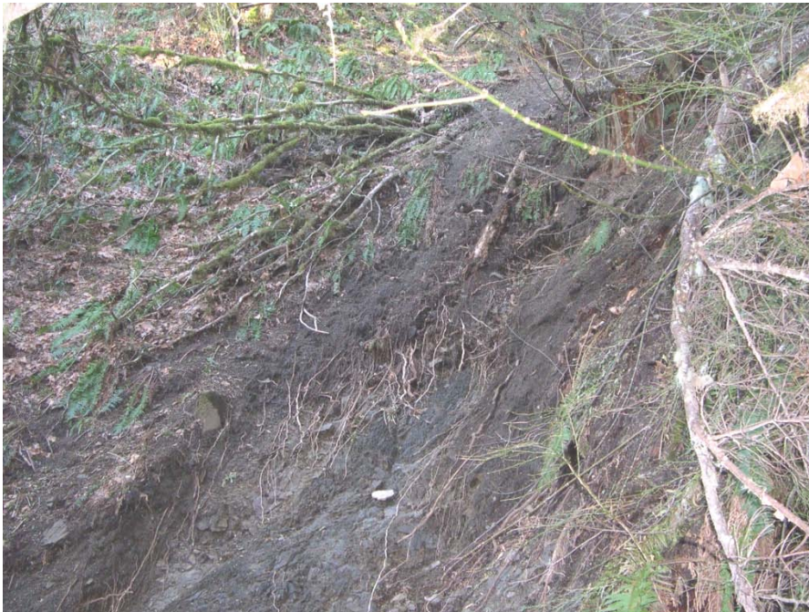
Figure 4 PI of 3810 NR site debris slide (Fitch). Photograph taken in Spring 2009. View looking northeast. (Photo by C. Hanell)
