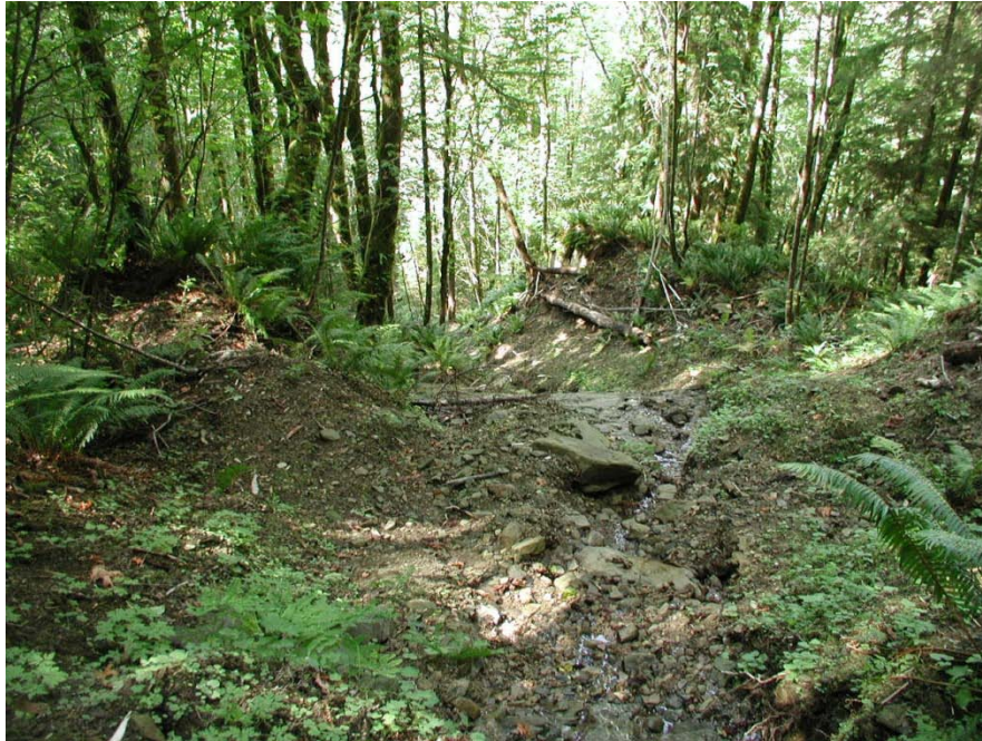
Figure 12 Scour along mid-reach of debris-flow track of 3830 NR site debris slide. Photograph take fall of 2009. View looking northwest. (Photo by J. Coyle)
