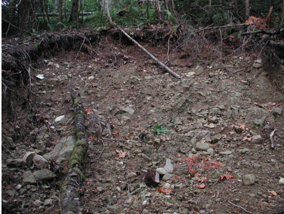
Figure 26 North PI of debris slides at NFR site (Kirkwood). Photograph taken Fall 2009. View looking east. (Photo by J. Coyle)
