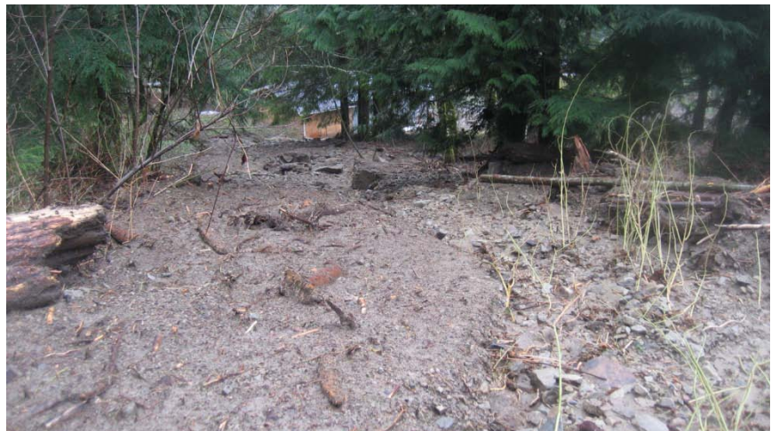
Figure 13 Debris on slope above garage/workshop at 3830 NR site. East corner of building can be seen in distance, with debris pointed toward corner. Photograph taken in early January 2009. View looking northwest. (Photo by D. Hooks)
