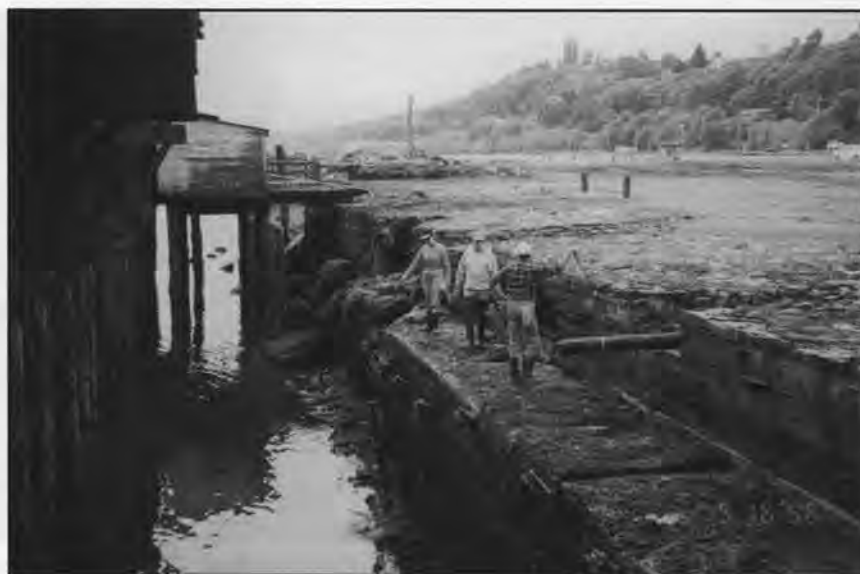
Figure 5. The central loading dock area near sample site 9 showing vertical walls of slag poured to form the seawall.
